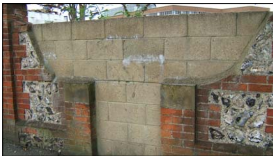
Fig. 26: Inappropriate filling of access point
