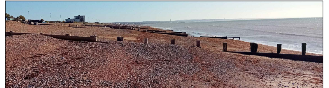
Photo of the same groyne two months after the works were completed
