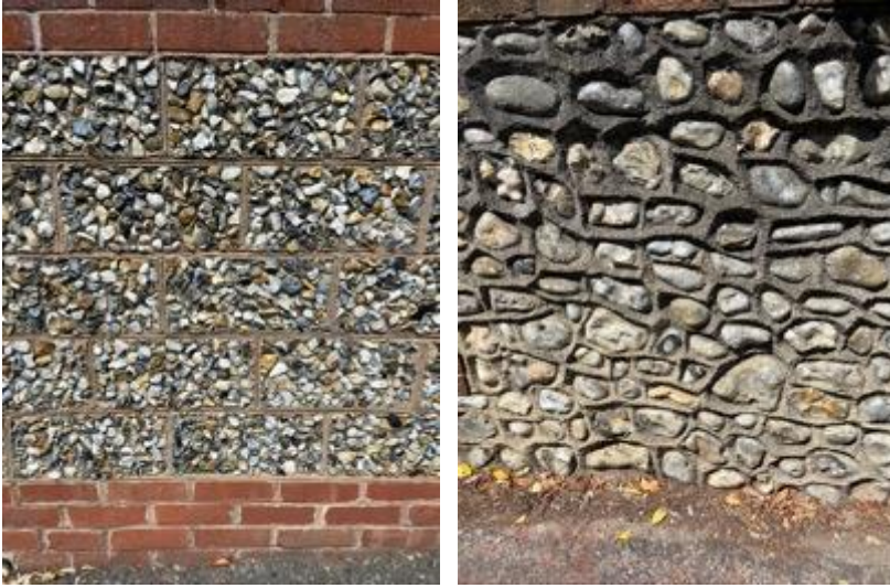
Fig 41: Modern inappropriate flint wall and poorly repaired historic wall
