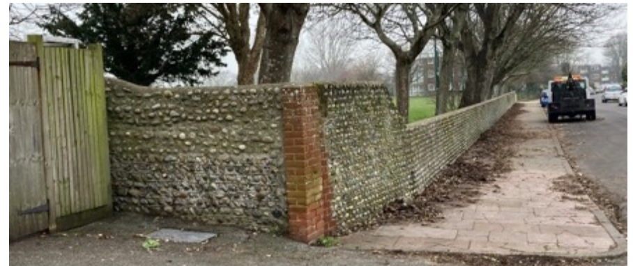
Figure 17: Flint wall to the north of The Bull's Head within the conservation area.
