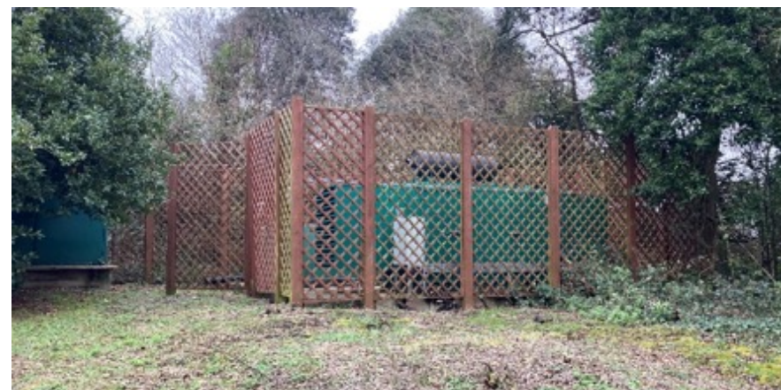
Figure 28: Plant within the grounds of Goring Hall
