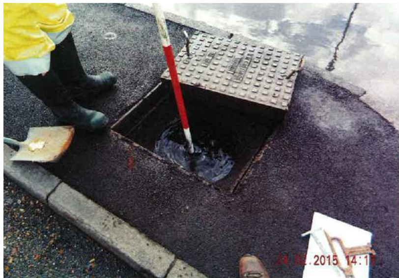
Figure 8-2 Photo of soakaway near the shops on The Broadway
